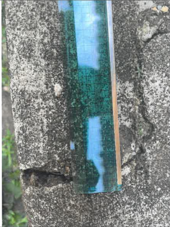
Photo G308-31: Wide Crack
