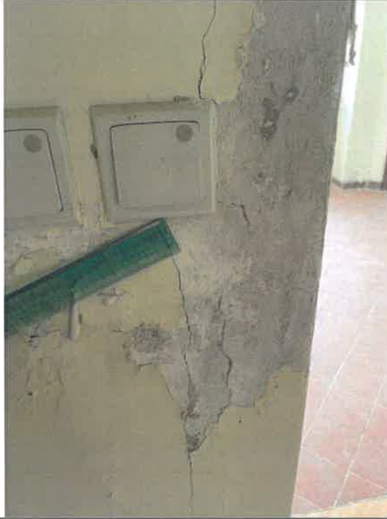
Photo: G303-37: Fine Crack on Surface
