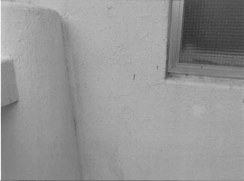
Photo: HKT03-53 Fine cracks on surface
