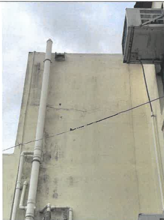
Photo: G303-42: Moderate Crack on Surface
