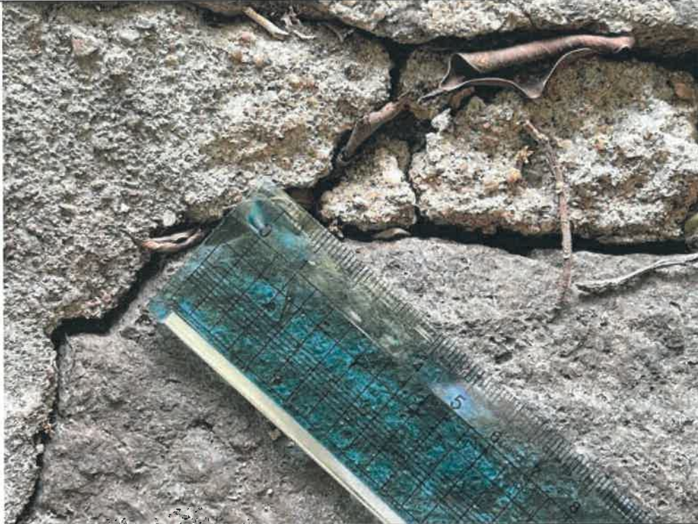
Photo : G202-11 Wide Crack on Surface
