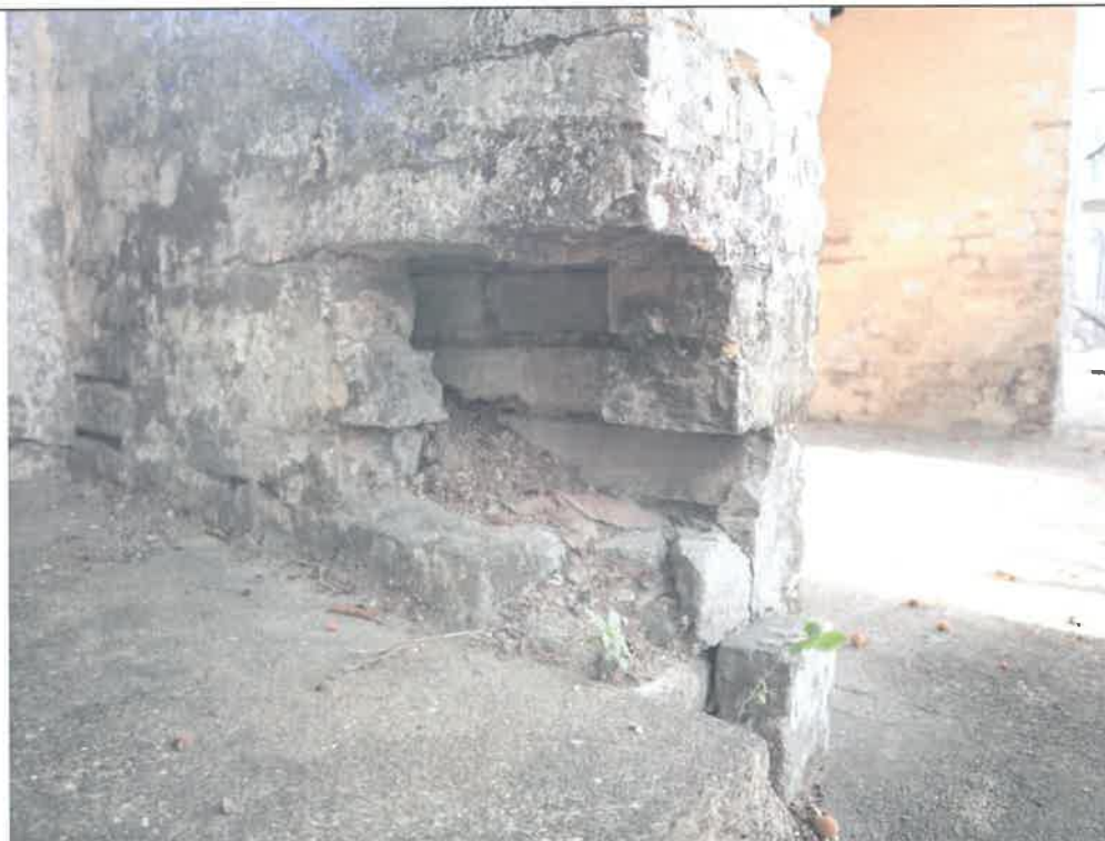
Photo 1-EG-10 Missing bricks on the structure
