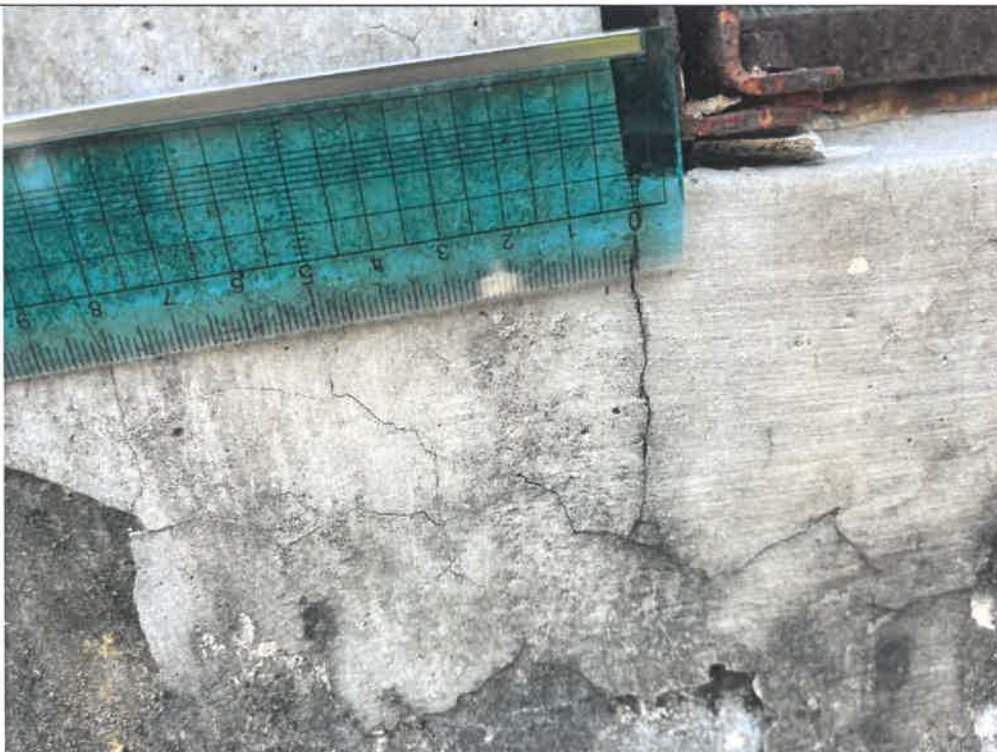
Photo G308-28: Moderate Crack
