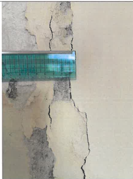
Photo: G303-38: Fine Crack on Surface
