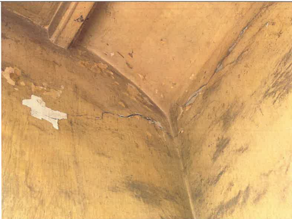
Photo G308-36: Moderate Crack on Surface
