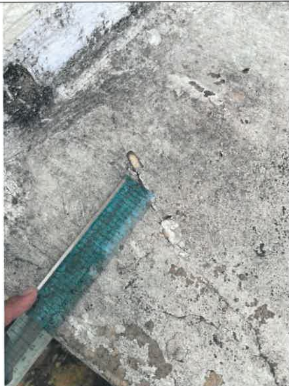
Photo: G303-36: Fine Crack on Surface
