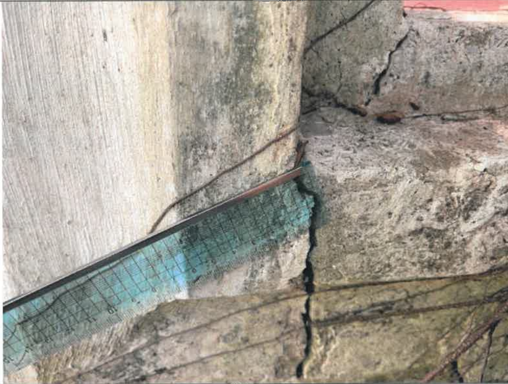
Photo : G202-15 Wide Crack on Surface
