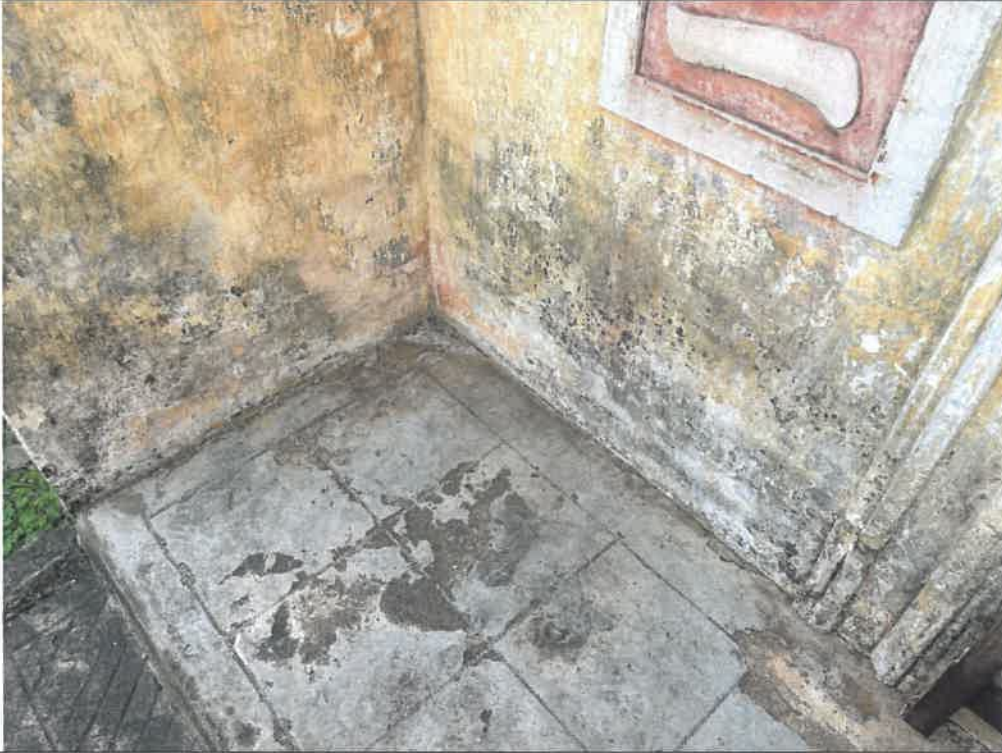
Photo G308-35: Moderate Crack
