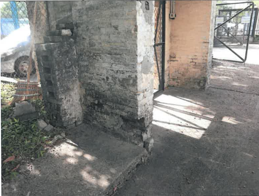
Photo 1- EG-9: Missing bricks on the structure
