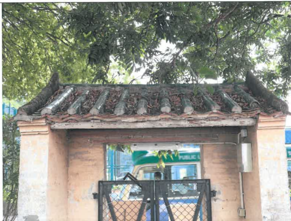
Photo 1- EG-6 Top tiles of the entrance gate
