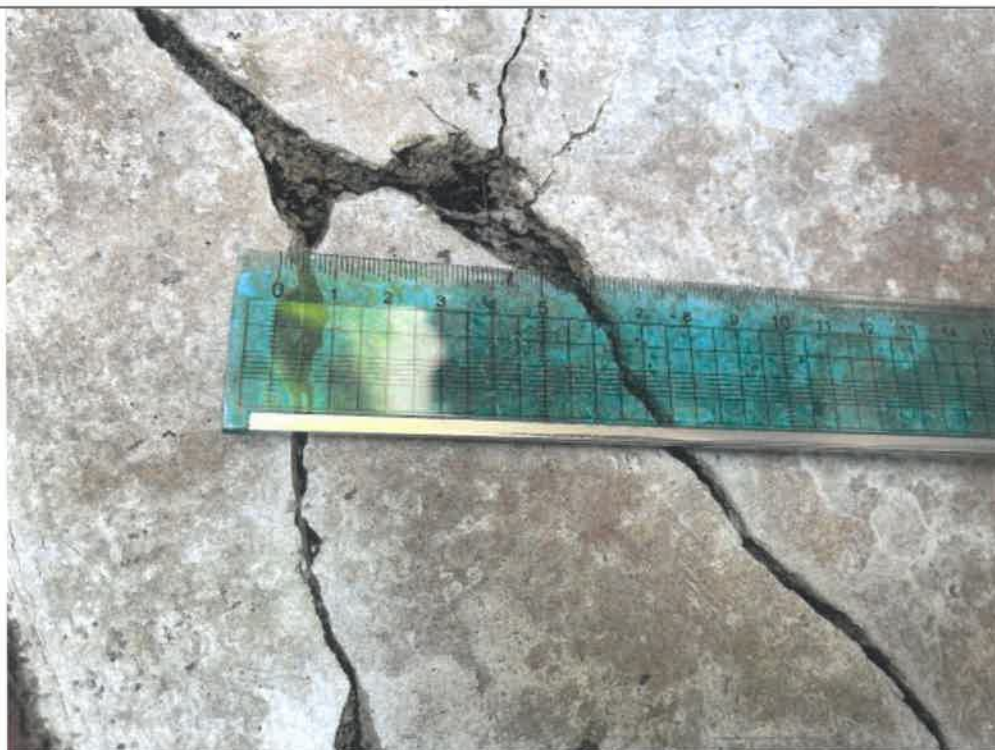
Photo : G202-14 Wide Crack on Surface
