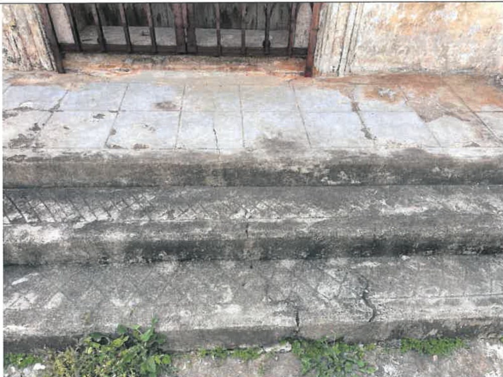
Photo G308-34: Wide Crack
