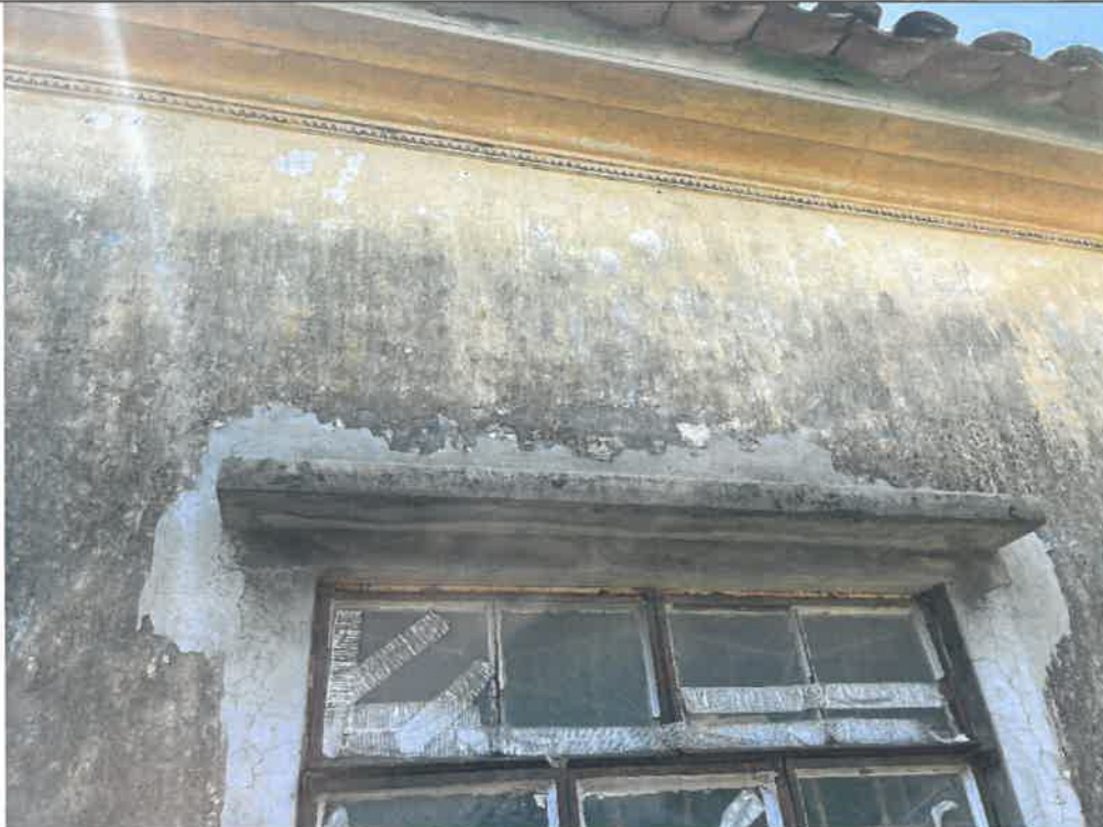
Photo G308-43: Moderate Crack
