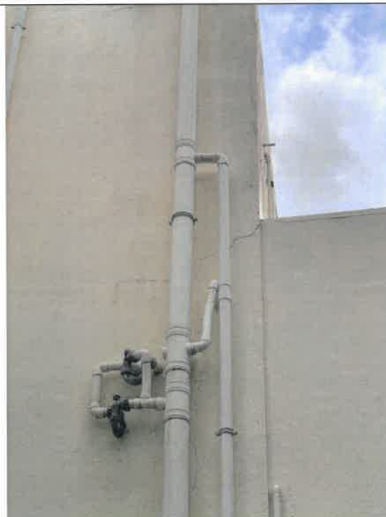
Photo: G303-40: Moderate Crack on Surface
