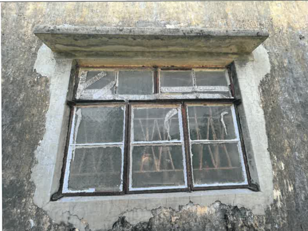
Photo G308-9: Orientation: (East to West), A Window Is located next to the room above left
