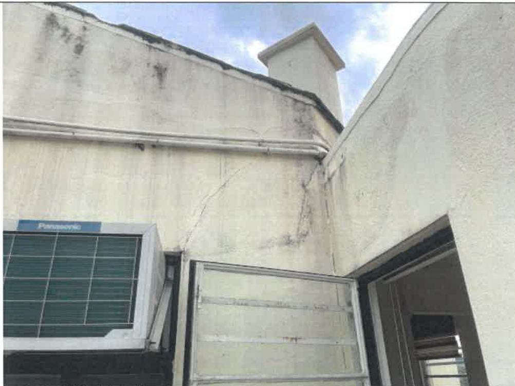
Photo: G303-34: Fine Crack on Surface
