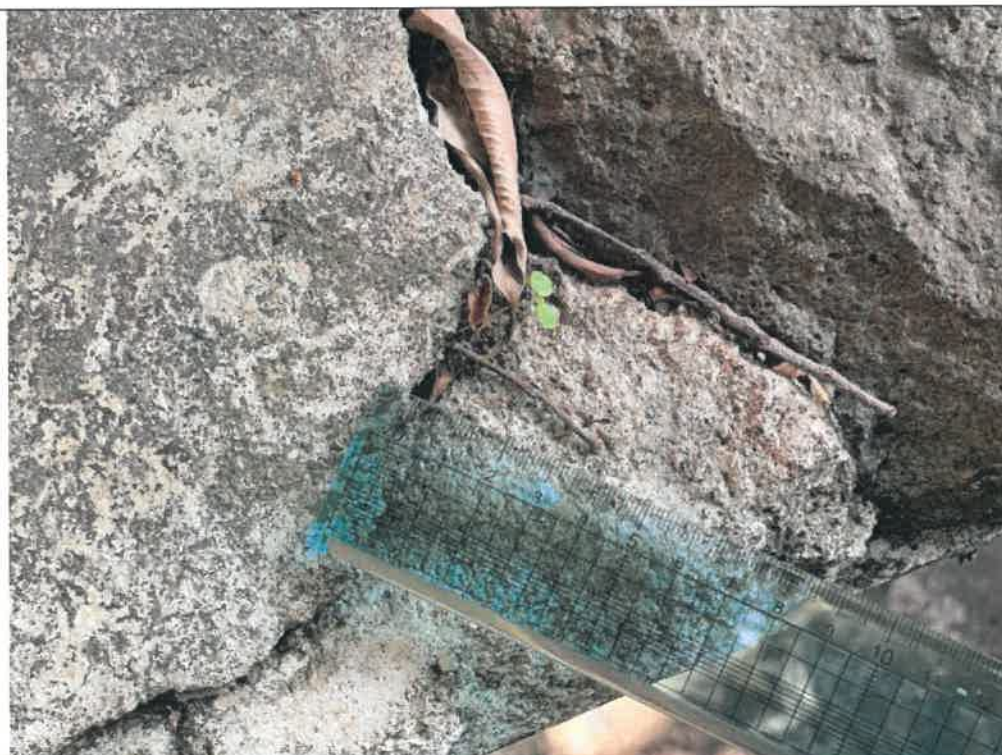
Photo : G202-12 Wide Crack on Surface
