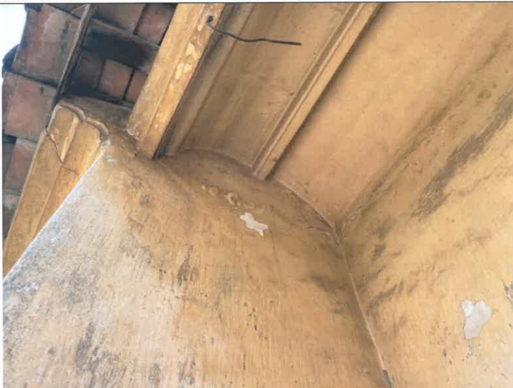
Photo G308-37: Moderate Crack
