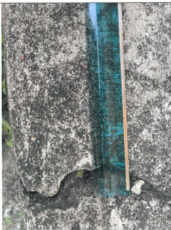
Photo G308-30: Wide Crack
