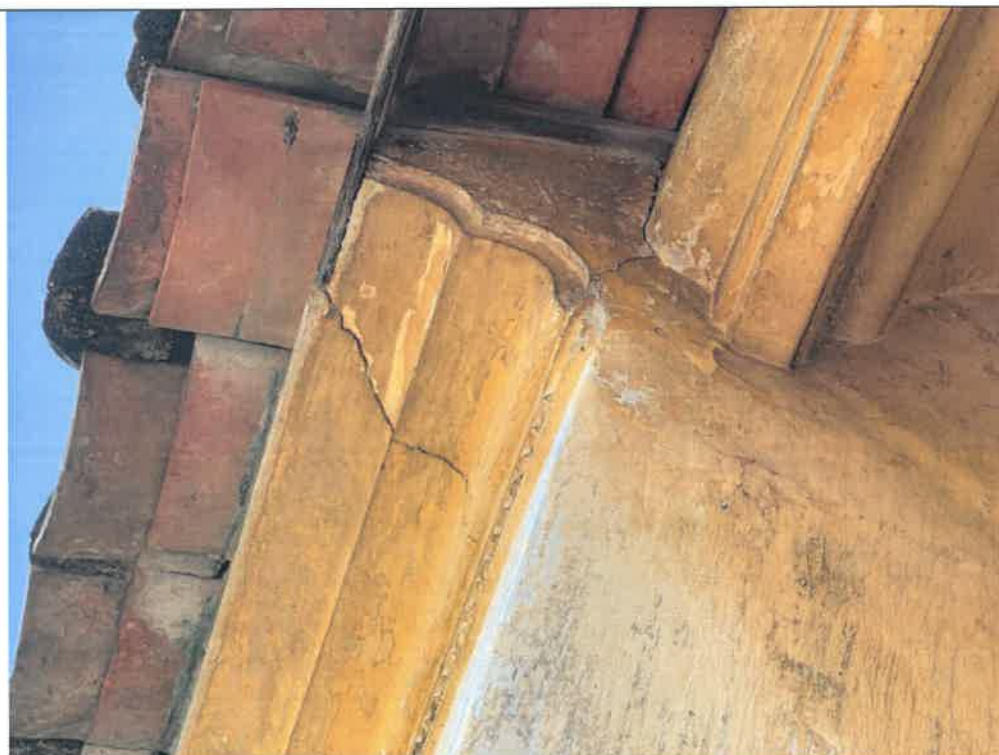
Photo G308-38: Wide Crack
