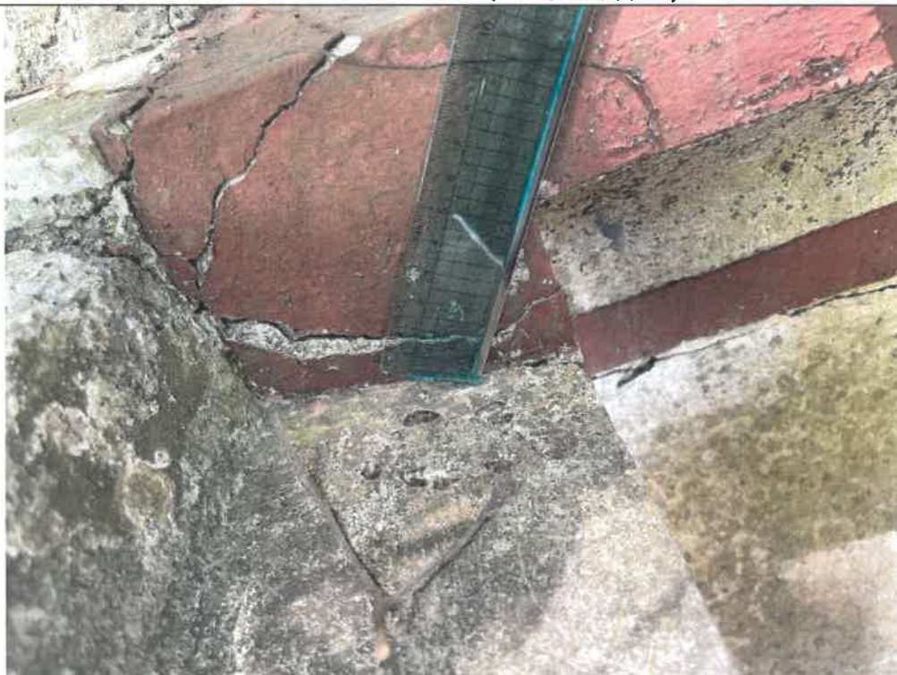
Photo : G202-13 Wide Crack on Surface
