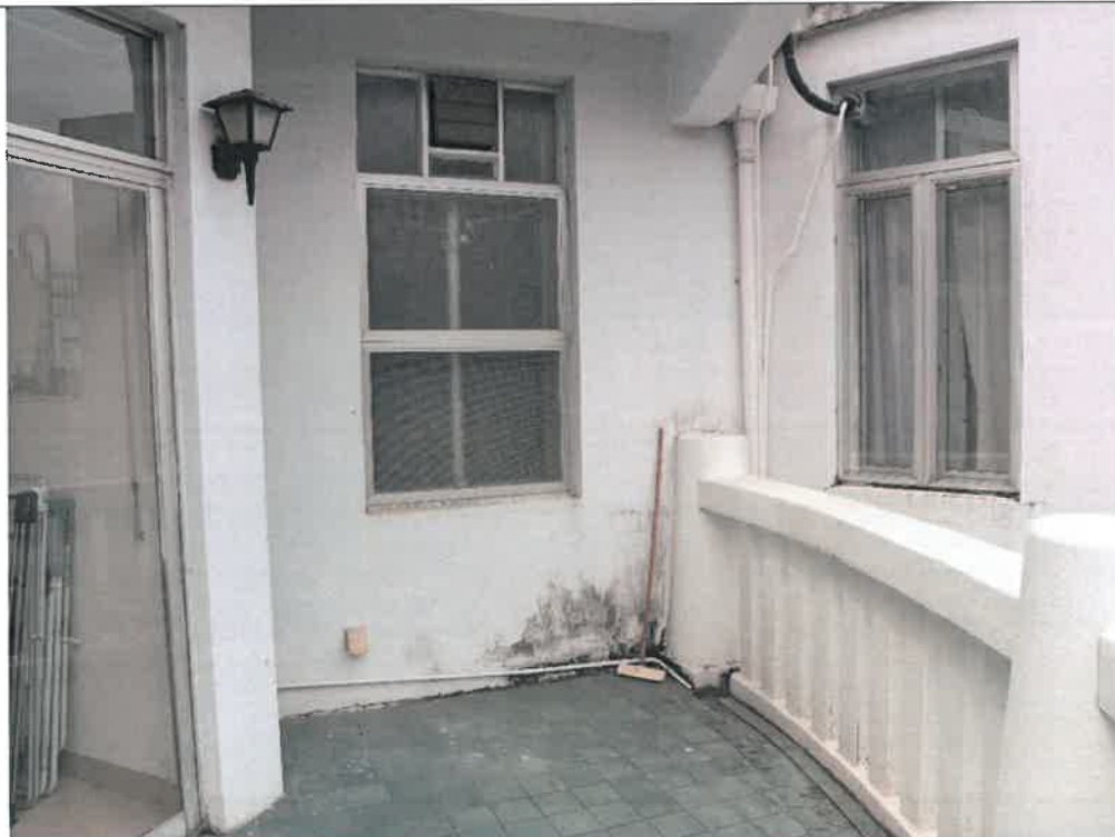
Photo: HKT03-52 Fine cracks on surface
