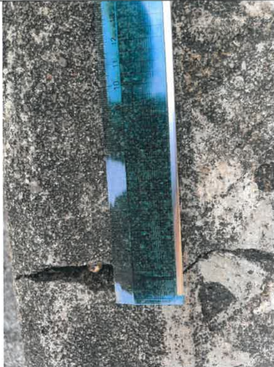
Photo G308-33: Wide Crack
