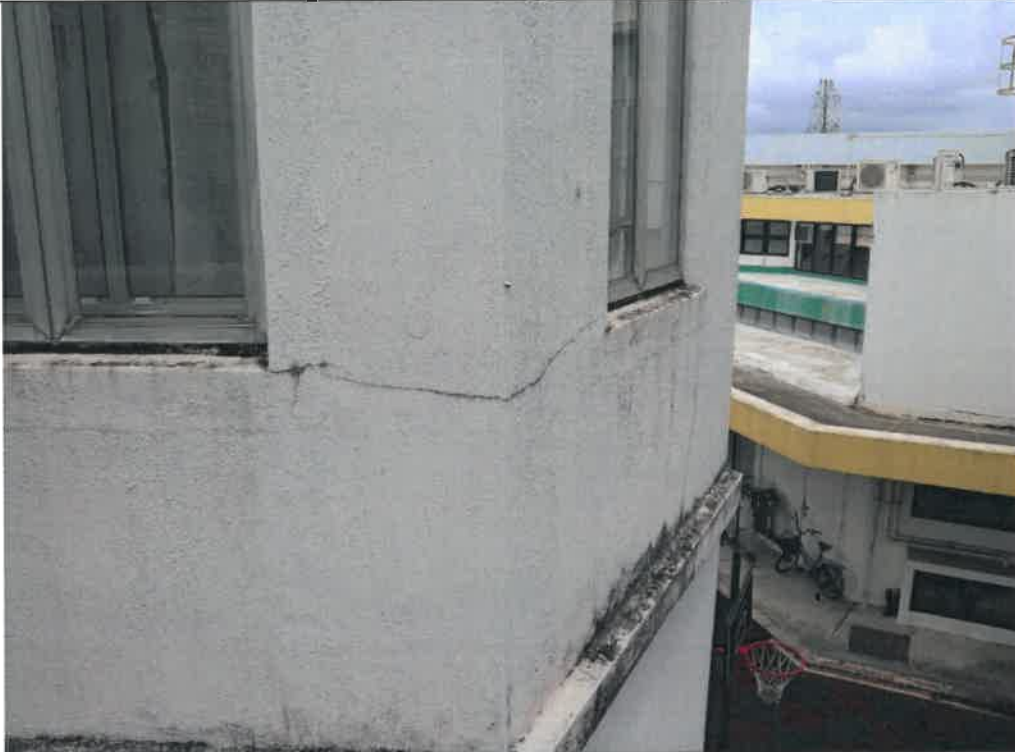
Photo: HKT03-51 Moderate cracks on surface
