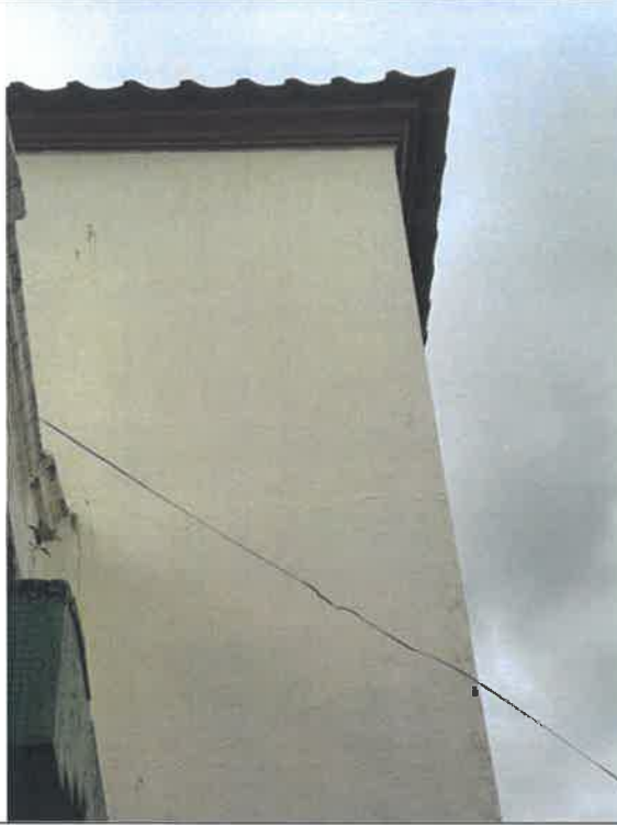
Photo: G303-41: Fine Crack on Surface
