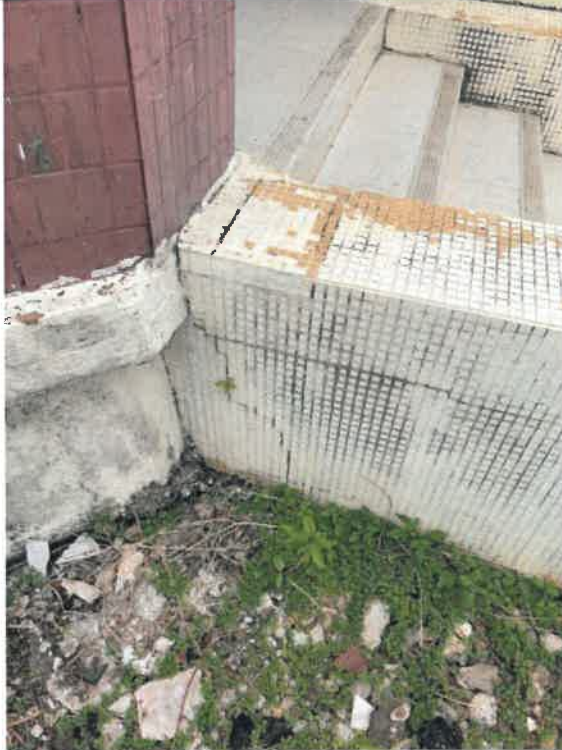
Photo: G303-39: Moderate Crack on Surface
