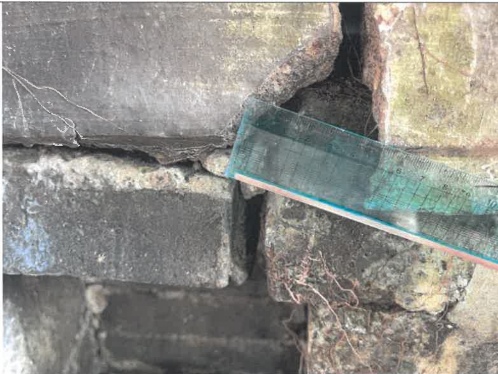
Photo : G202-18 Wide Crack on Surface
