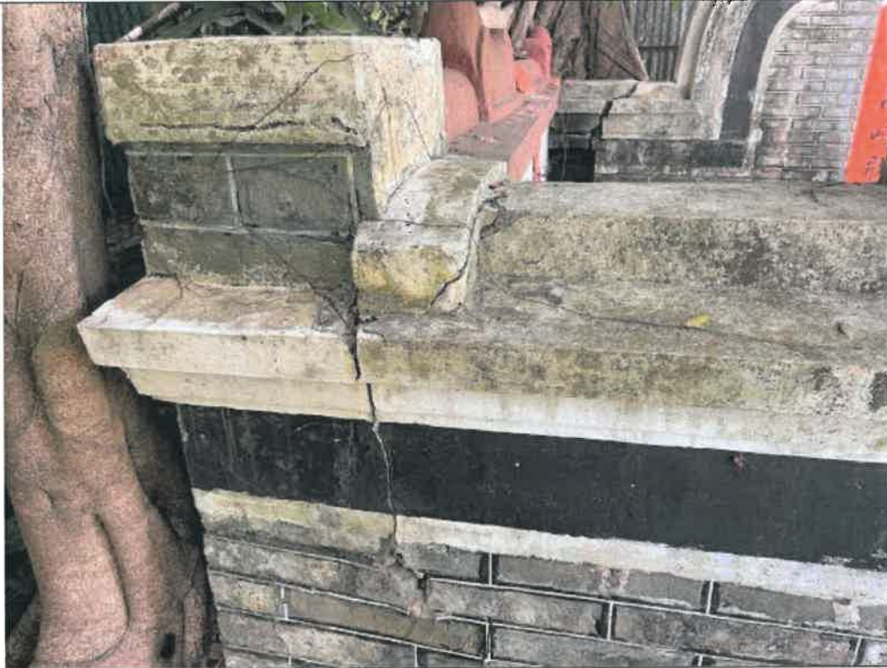
Photo : G202-19 Moderate Crack on Surface
