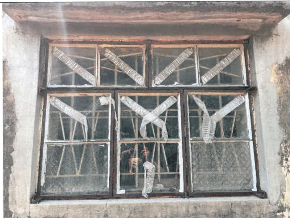
Photo G308-10: Orientation: (East to West), A Window Is located next to the room above right
