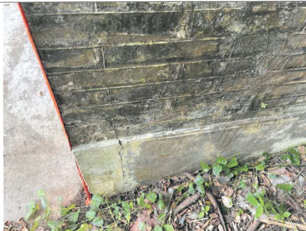
Photo : G202-16 Fine Crack on Surface
