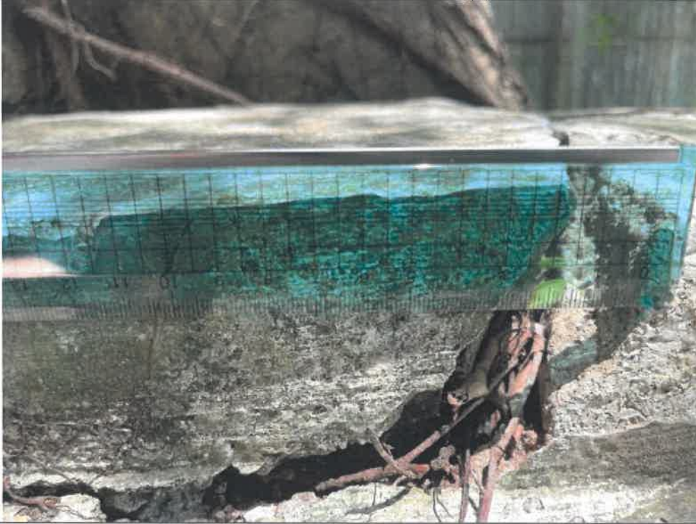
Photo : G202-17 Wide Crack on Surface
