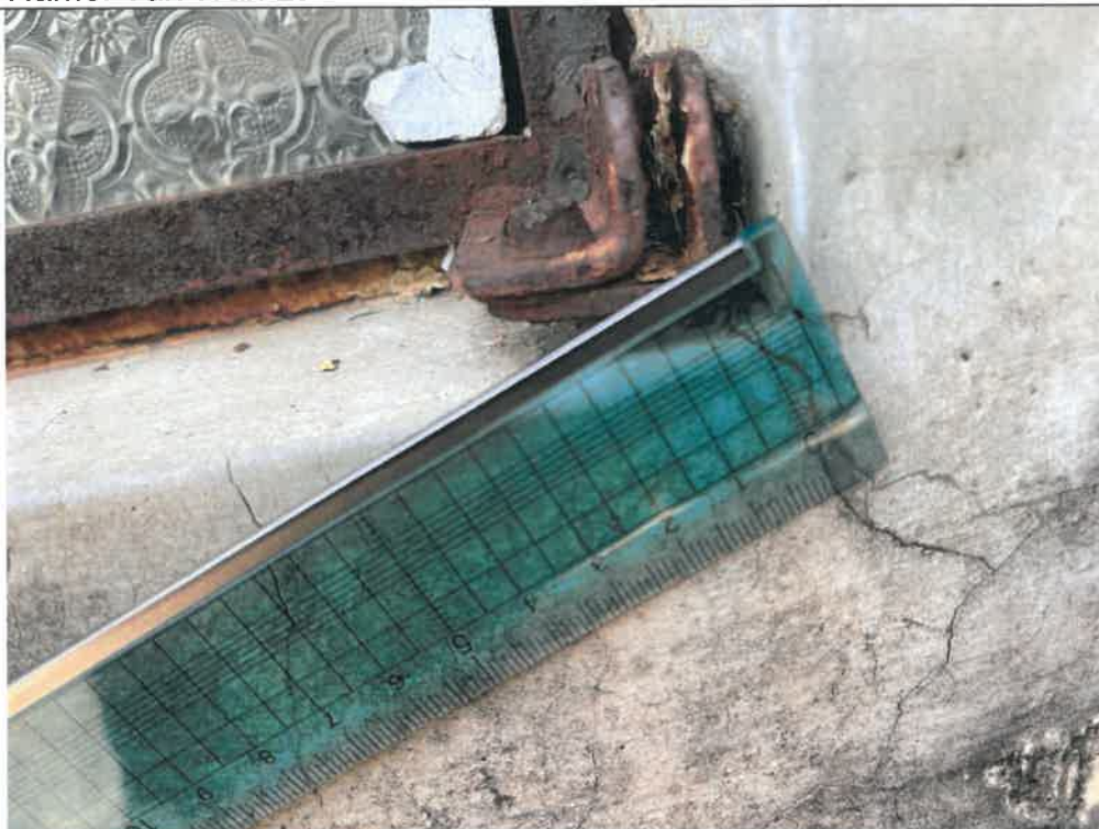
Photo G308-29: Moderate Crack
