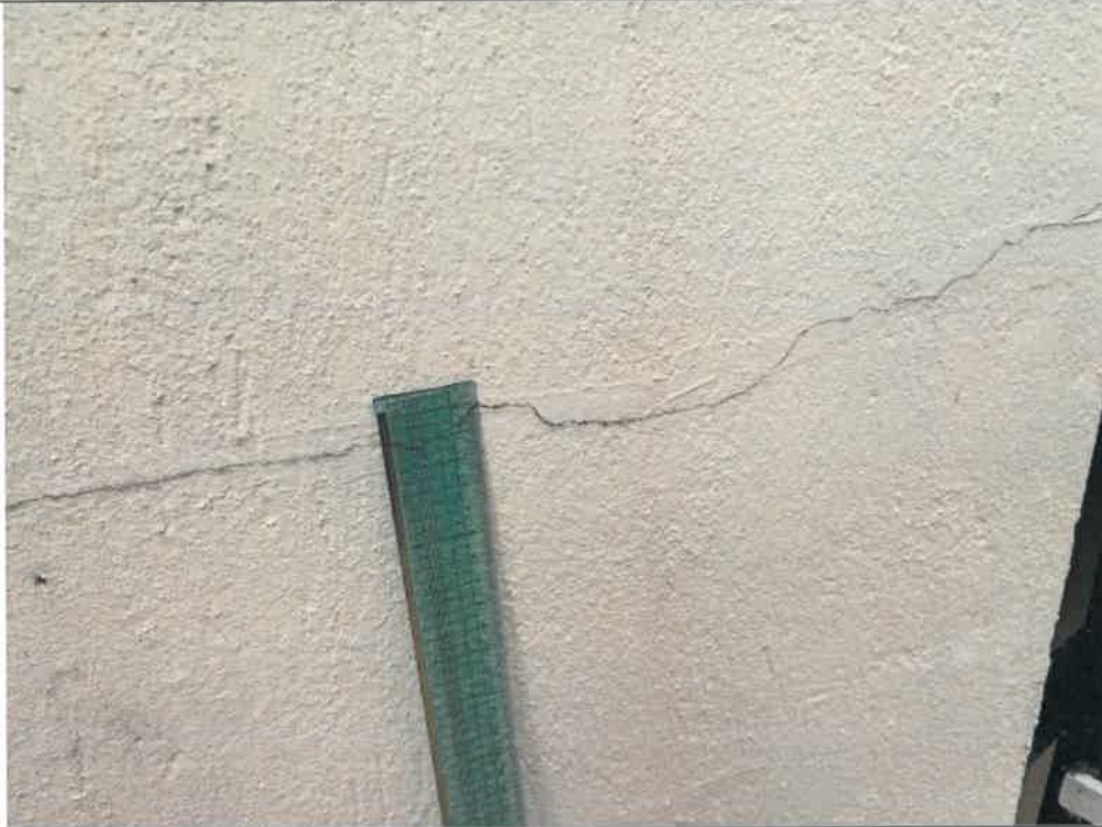
Photo: G303-35: Fine Crack on Surface
