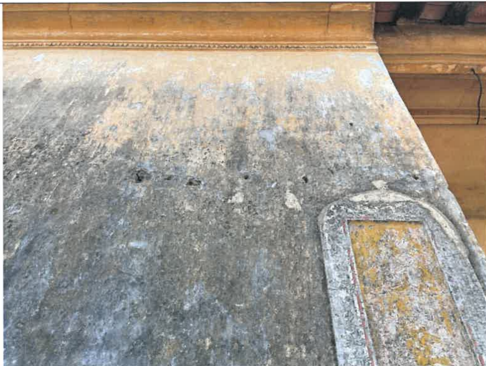
Photo G308-42: Moderate Crack
