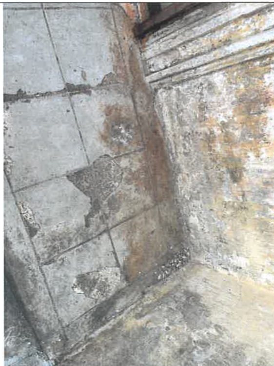
Photo G308-40: Wide Crack
