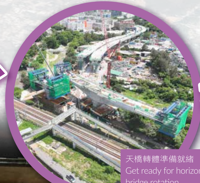
於鐵路非行車時間安裝掛籃式模板，以建造橋面 Installation of form traveller for bridge deck construction during non-traffic hours of the railway line
